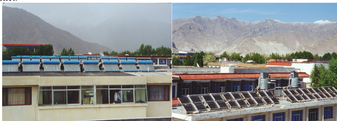
Fig. 2 Application of solar water heater in Tibet
