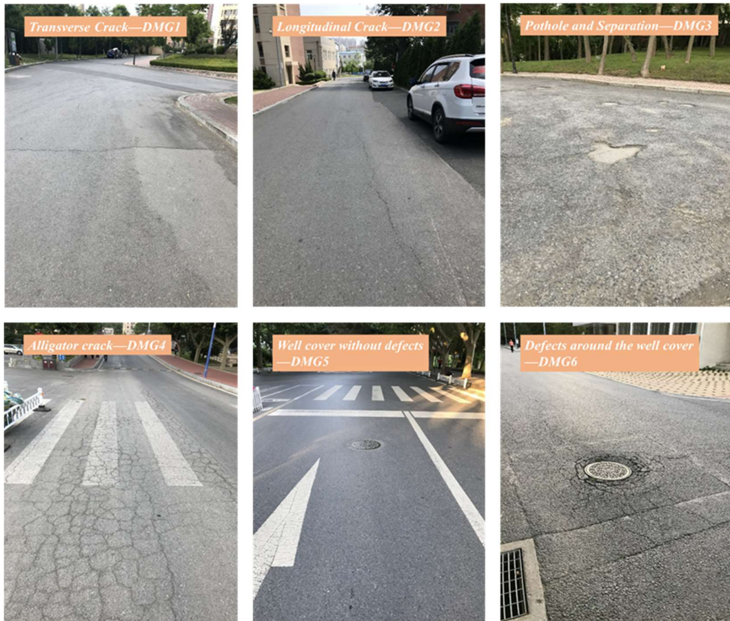
Figure 1. Road pavement damage images
