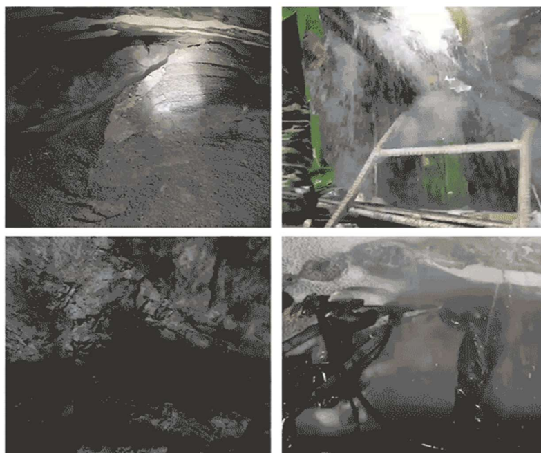
Fig.6 Water and sand inrush in tunnel
