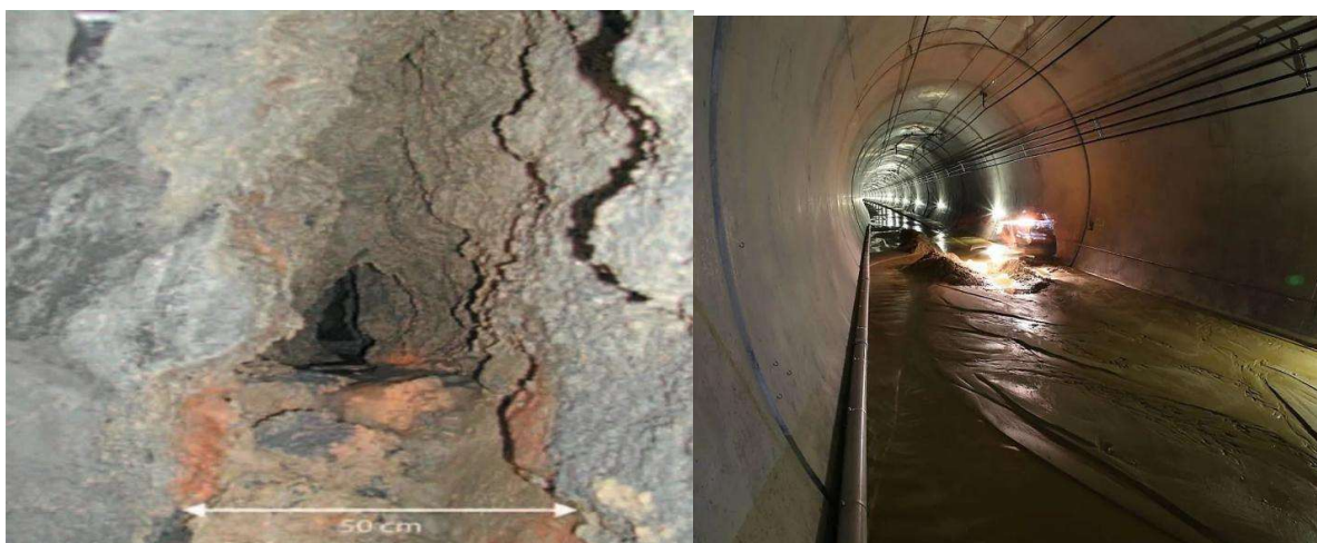
Fig.4 Water inrush at Leche Hill base tunnel
