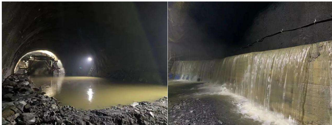
Fig.8 Site of water gushing in Jixin Tunnel
